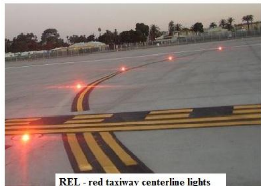
Figure 3: Runway Entrance Lights
